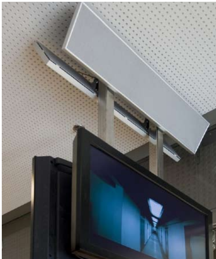
Figure 10. Panphonics Sound Shower speaker installed with digital signage
